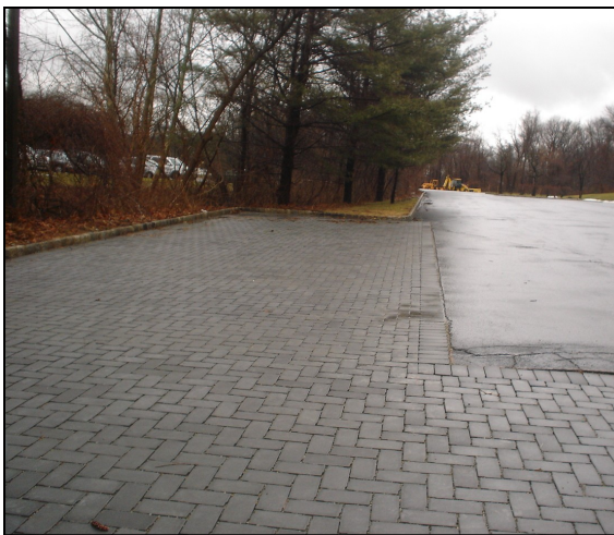
Pervious pavement on this Normandy Property Office Complex parking lot infiltrates stormwater that would have been runoff. See Troy Brook RSMP, pg.3 Photo by Pat Rector
