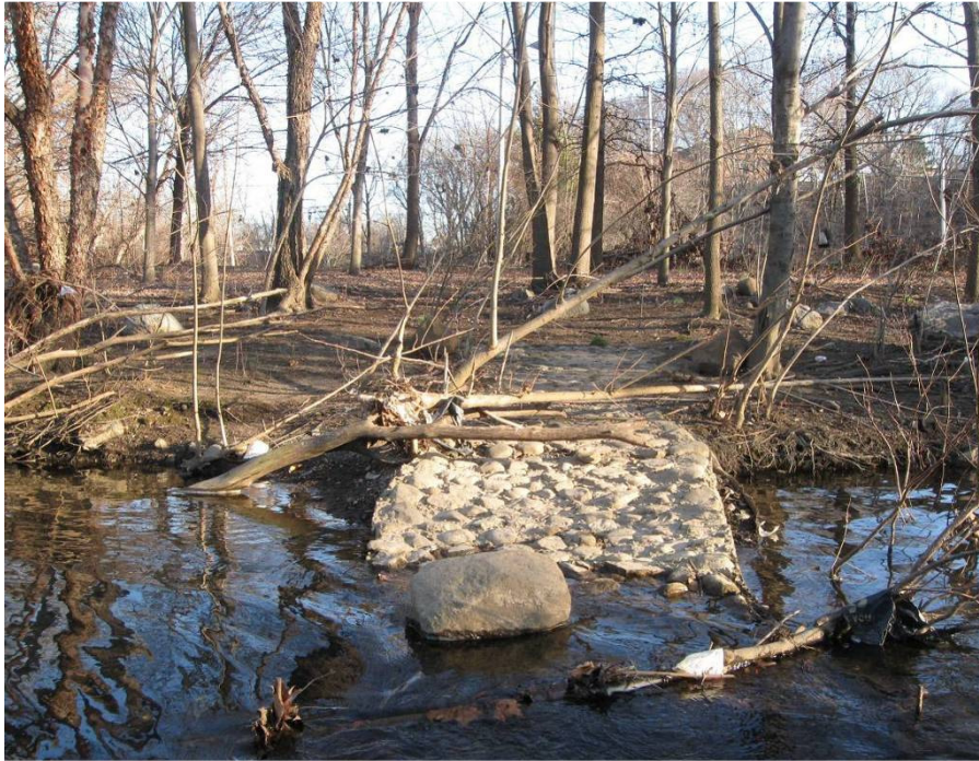
Figure 20: Area of Concern #4 Concrete and Stone Ramp
