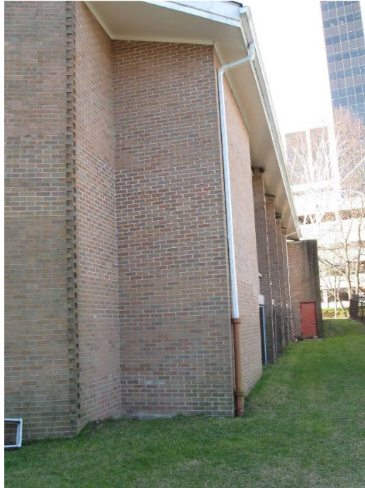
Figure 11: Area of Concern #3 Eastern Corner of the Church
