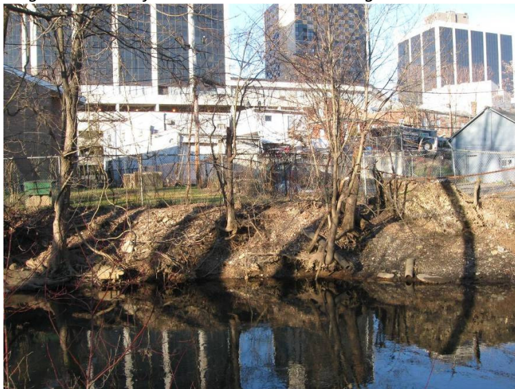
Figure 9: Area of Concern #2 Fences Leaning into the Stream
